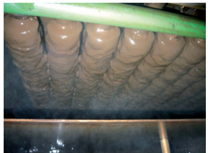
Particles and sludge attached to the magnetic separator (Photo: BFI)
