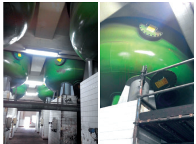
WTP industrial sand filters (Photos: AcelorMittal)
